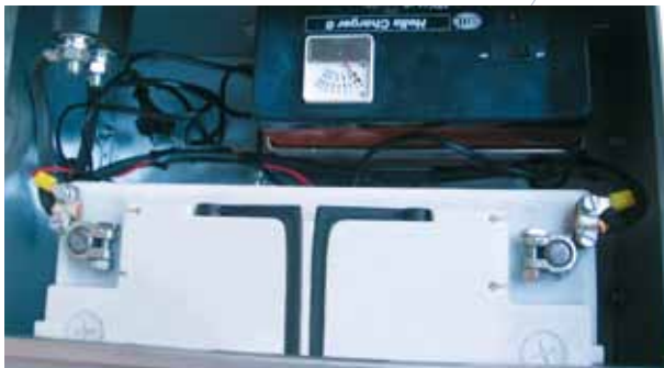
Battery with charger (230 volt).
