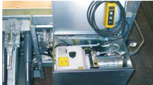
Electrical pump with control unit.
